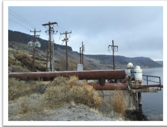
Existing Intake Structure and Pump Station at CJ Strike Reservoir, Operated by Simplot Corporation
